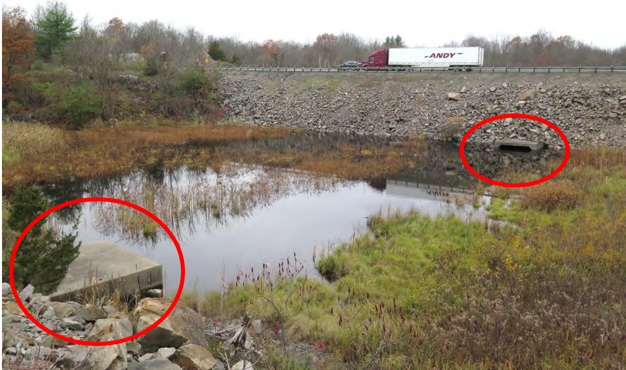
Figure 19: Photo of flooded box culverts (circled in red) on Highway 401 between Highway 137 and Escott-Rockport Road.
