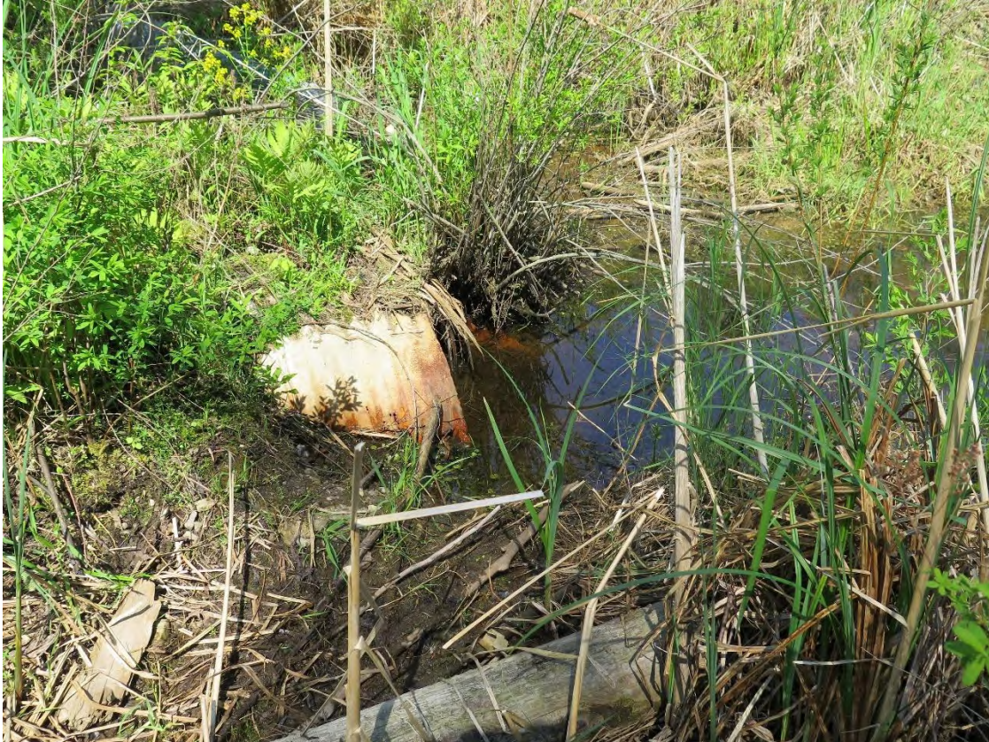
Figure 27: Photo of the undersized culvert on County Road 2 within the Jones Creek pathway.
