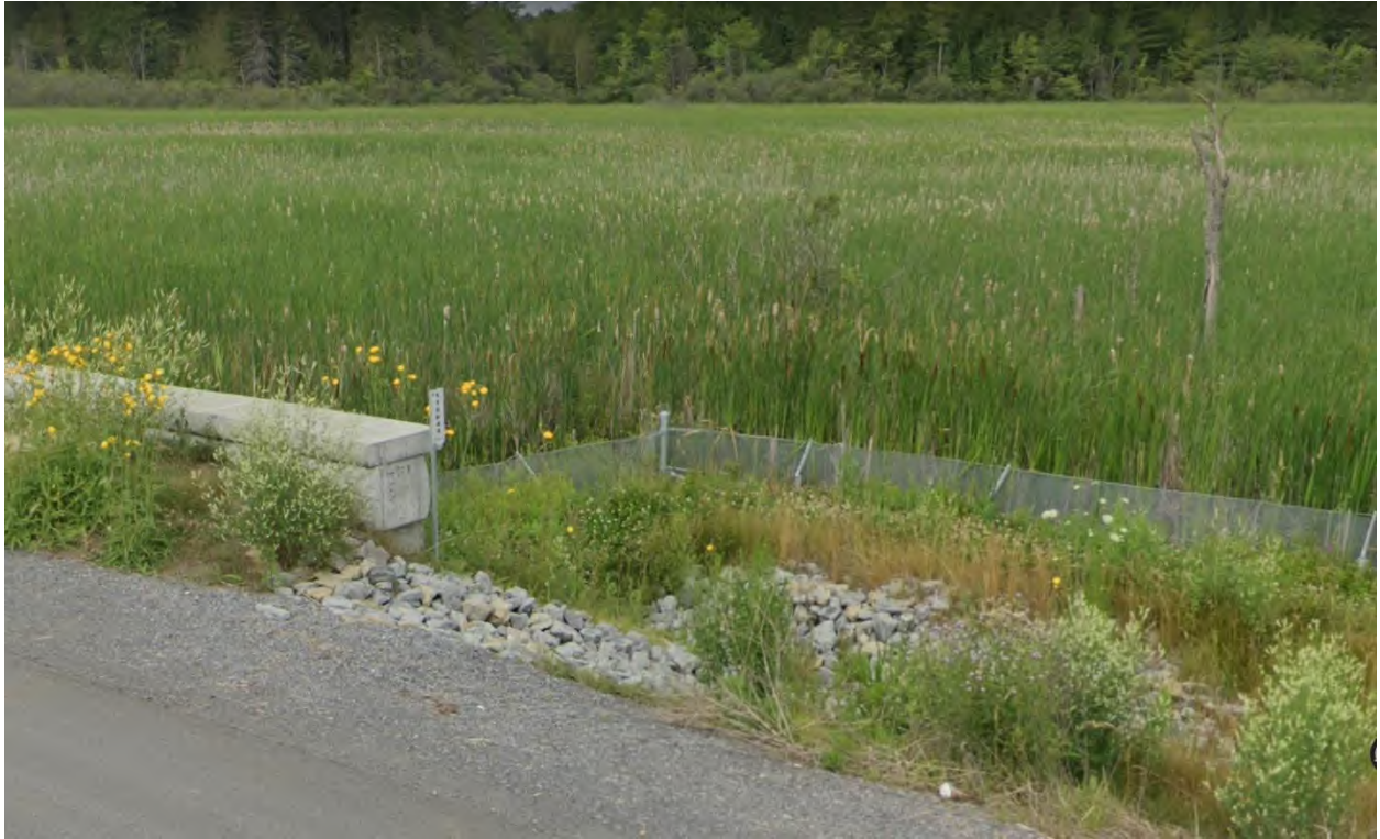
Figure F2: Two-metre-tall wildlife exclusion fence (hardwire mesh and metal poles) with overhang tied into concrete wildlife barrier along wetland habitat in Ottawa (© K. Black).
