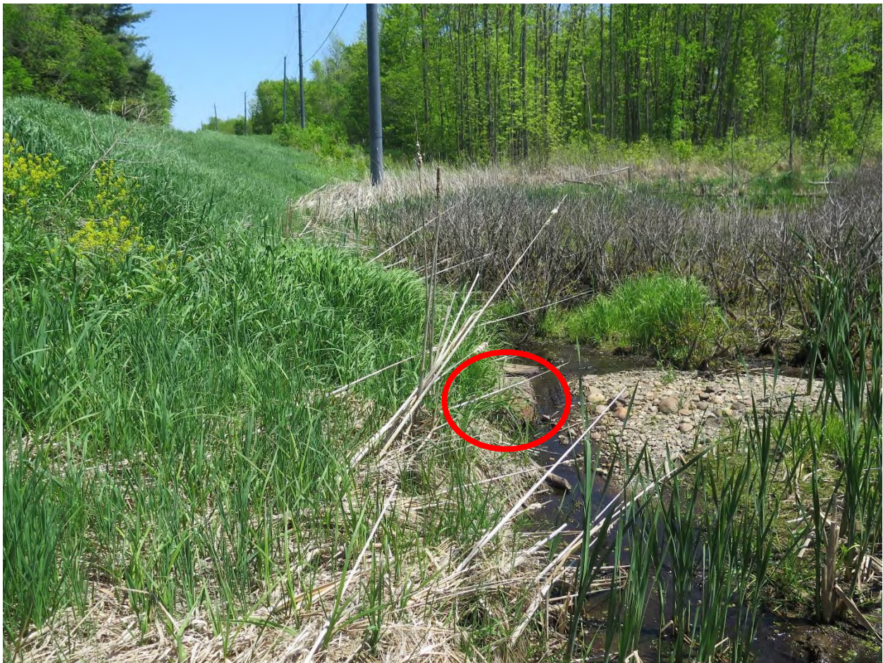
Figure 21: Photo of the undersized culvert on County Road 2 within the Rockport to Waterton pathway.
